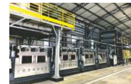
Pad Steam / Washing Range
